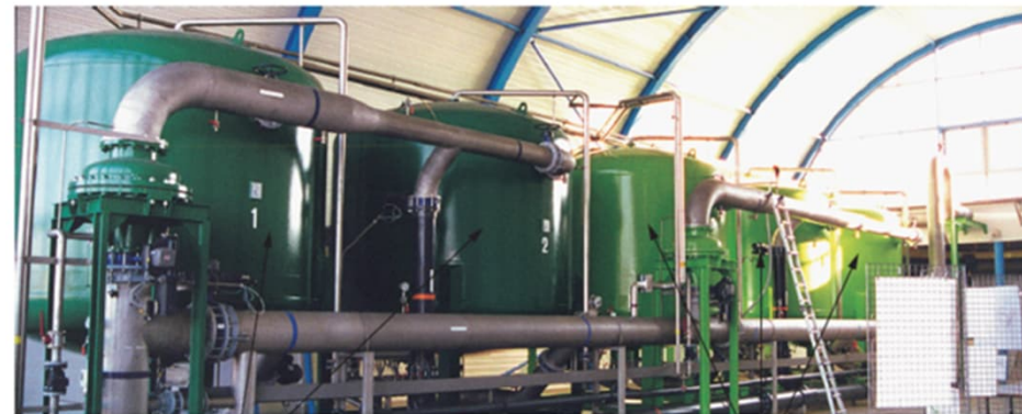
Raw water aeration
