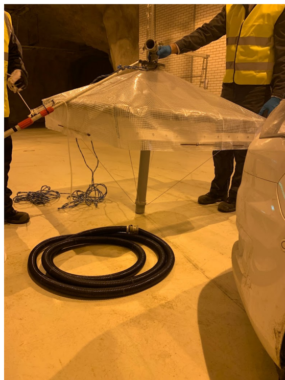
(b) Off-gas hood structure.
